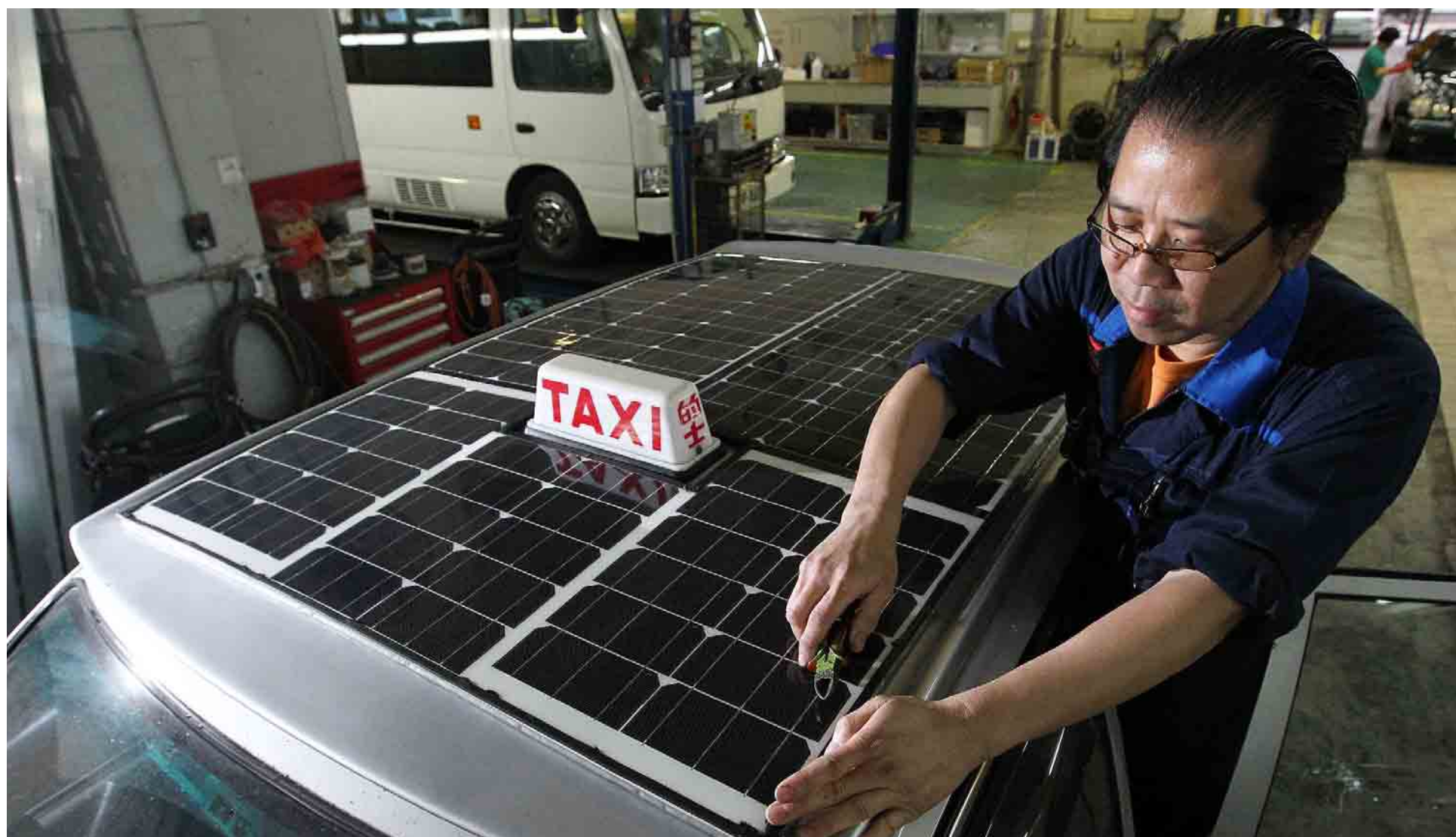
A taxi in Yuen Long is fitted with solar panels, integral to a new air-conditioning system made in Hong Kong. The panels convert solar power into electrical energy. Photo: May Tse
